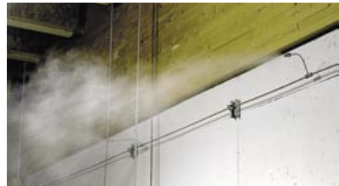
A humidity control system in operation
